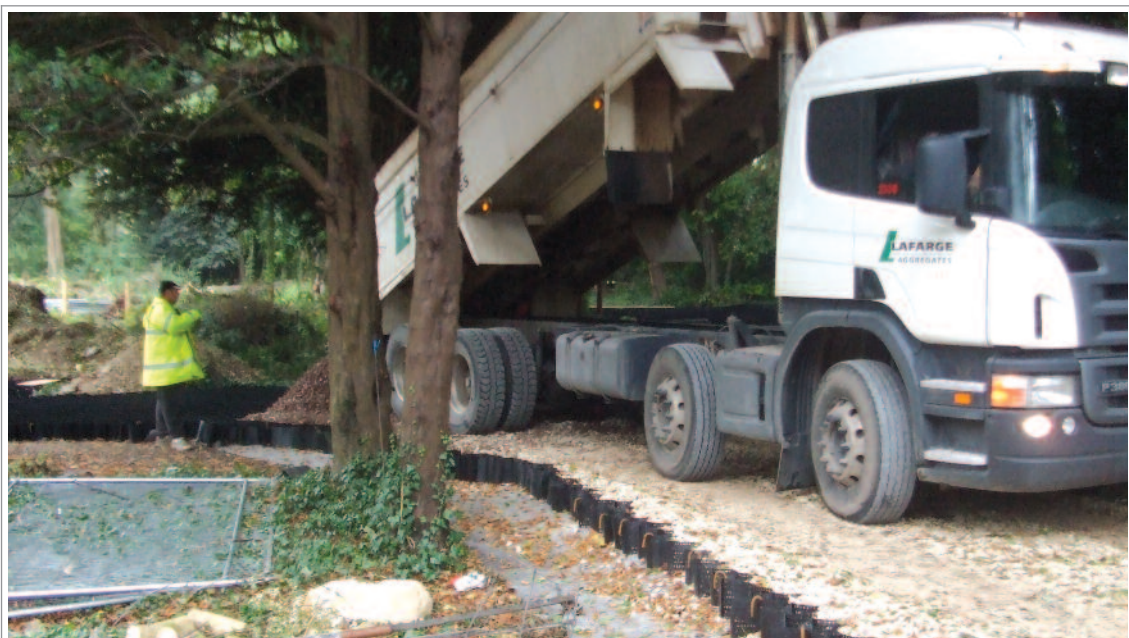
Installing a special surface to allow for heavy plant access through sensitive woodland during construction.
