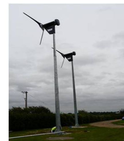
Figure 5.5: 2 x 6 kW Turbines at Leventhorpe school
