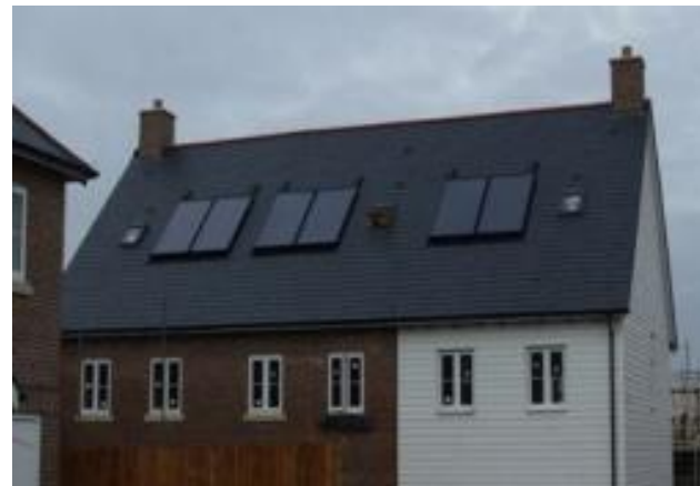
Figure C2 Solar hot water installation. Schuco flat plate system providing domestic hot water ( photo courtesy of Ecolution Renewables)
