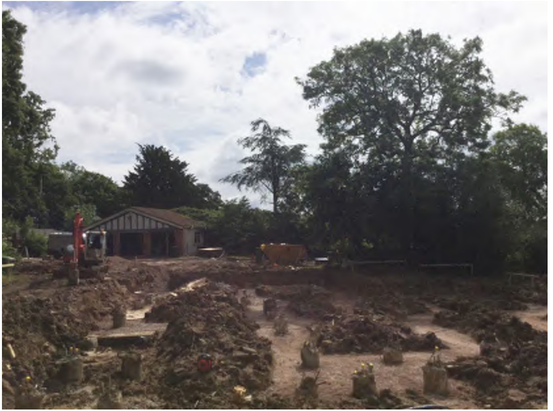
Photograph 1 Groundworks immediately to the south of Barnet Lane in the north of the parcel
