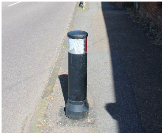
Figure 80 Plastic bollard on Blanche Lane
