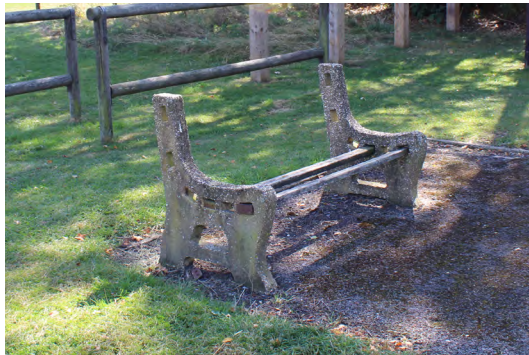
Figure 79 Damaged bench on Blanche Lane
