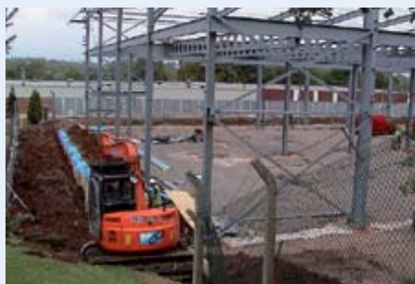
Stage 4: Make sure that the presence of the root barrier membrane is recorded and is not disrupted by future developments and landscaping.
