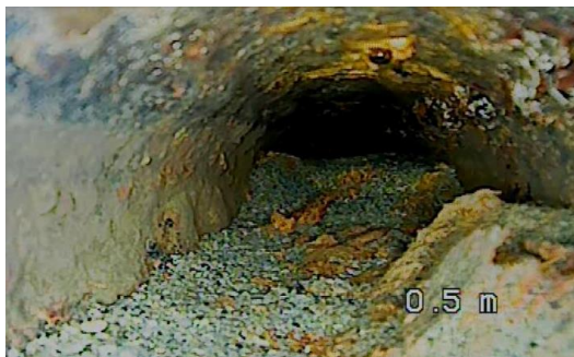
Figure 26: Sediment in pipework
