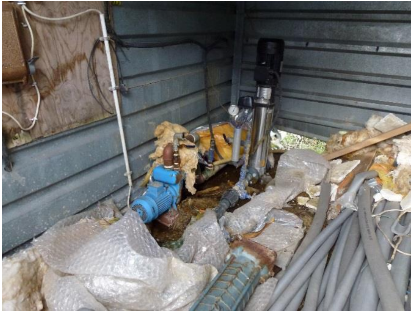
Figure 18: Distribution pipework before major corrective work
