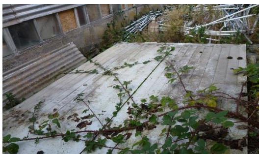
Figure 20 : Vegetation covering poorly constructed well cover
