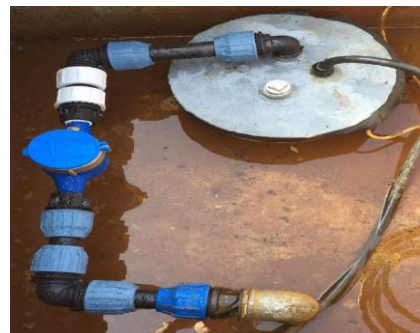
Figure 27: Poorly constructed headworks on source
