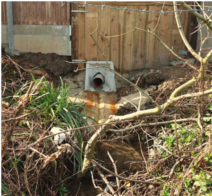
Figure 2.2 Outfall pipe from rear of No. 24 Wayside Road (Location shown circled in green in Figure 2.1)
