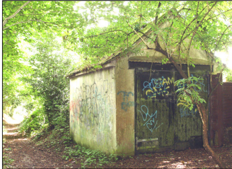
Figure 42. Graffiti on garage, Malt Lane
