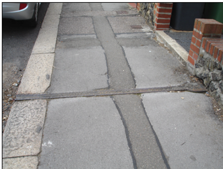
Figure 31. Character Zone 2: negative factor; tarmac tracks along Station Road
