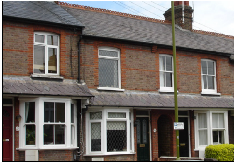
Figure 32. Station Road: various modern window styles contrasting with original timber sashes (right)
