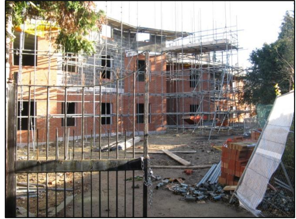
Figure 17 - The development of flats under construction, viewed from the Windmill Lane side.
