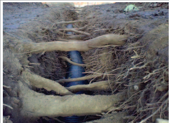
A section of drainage pipeline installed under tree roots following excavation using an air spade.
