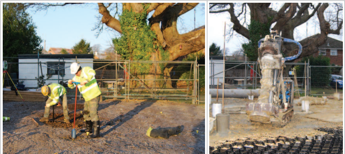
Using a hand auger to ensure proposed locations for piles do not conflict with tree roots within the root protection area of a veteran sweet chestnut tree. Note the BS 5837:2005 specification fencing in the background. The area was then covered with ground protection to allow a lightweight piling rig to work without damage to the underlying tree roots.
