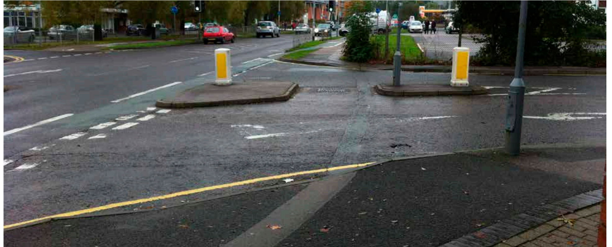
Figure 4 – Lack of tactile paving and dropped kerb facility at wide mouth of Elstree Way/Maxwell Road junction.
