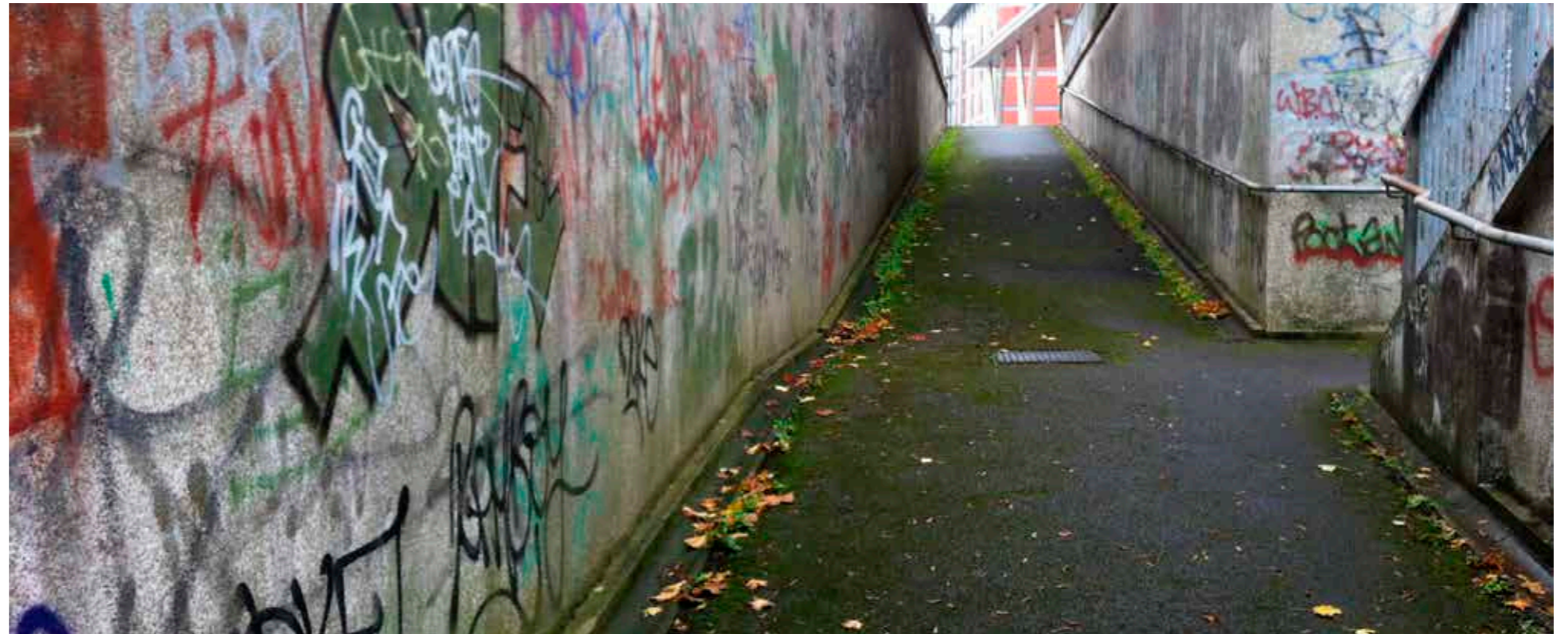
Figure 5 – Unattractive and uninviting existing pedestrian subway under Elstree Way (close to its junction with Bullhead Road) with lack of cyclist provision.
