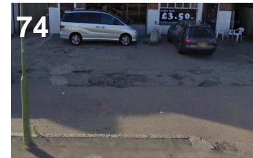
74. Private ownership of forecourts has led to lack of satisfactory maintenance of hard standing
