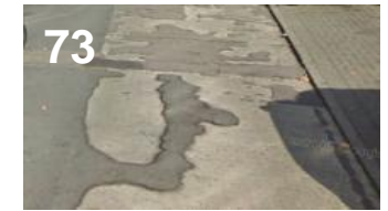
73. Poor carriageway surfaces
