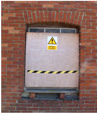
Figure 74 Boarded up window at 93 Blanche Lane
