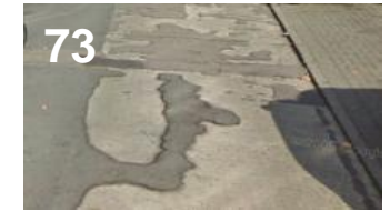
73. Poor carriageway surfaces
