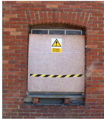
Figure 74 Boarded up window at 93 Blanche Lane
